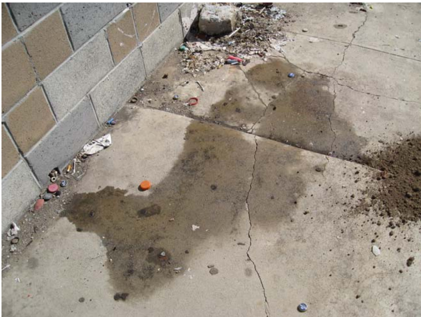
Stained concrete observed on the northern concrete paved portion of the Property.
